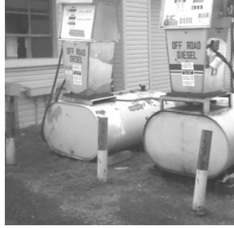
What's wrong with this picture?
