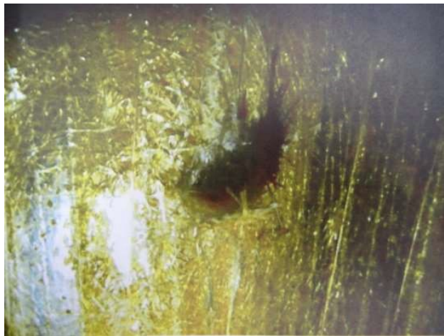
ASTSWMO Case summary #20: UST fibers exposed due to chemical exposure (FRP)
