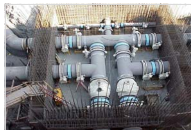
60 inch pipe in valve vault
