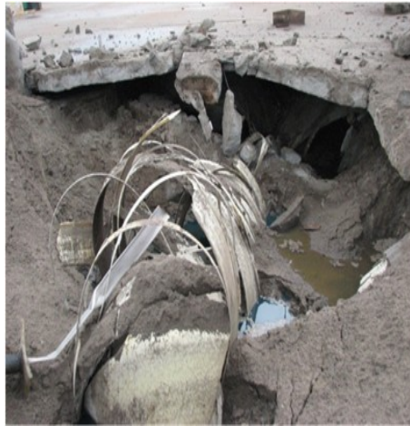
Steel is naturally grounded. A steel tank won't explode like this FRP tank did when lightning struck nearby.
